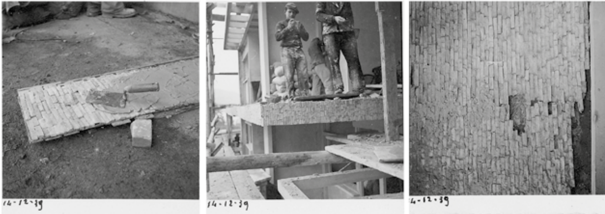
Figures 8a-c. Laying of the cladding with marble splits. AGT, photographs, 72/043/C/S, GF043C - 72/040/C/S, GF040C - 72/041/C/S, GF041C, 14/12/1939).
