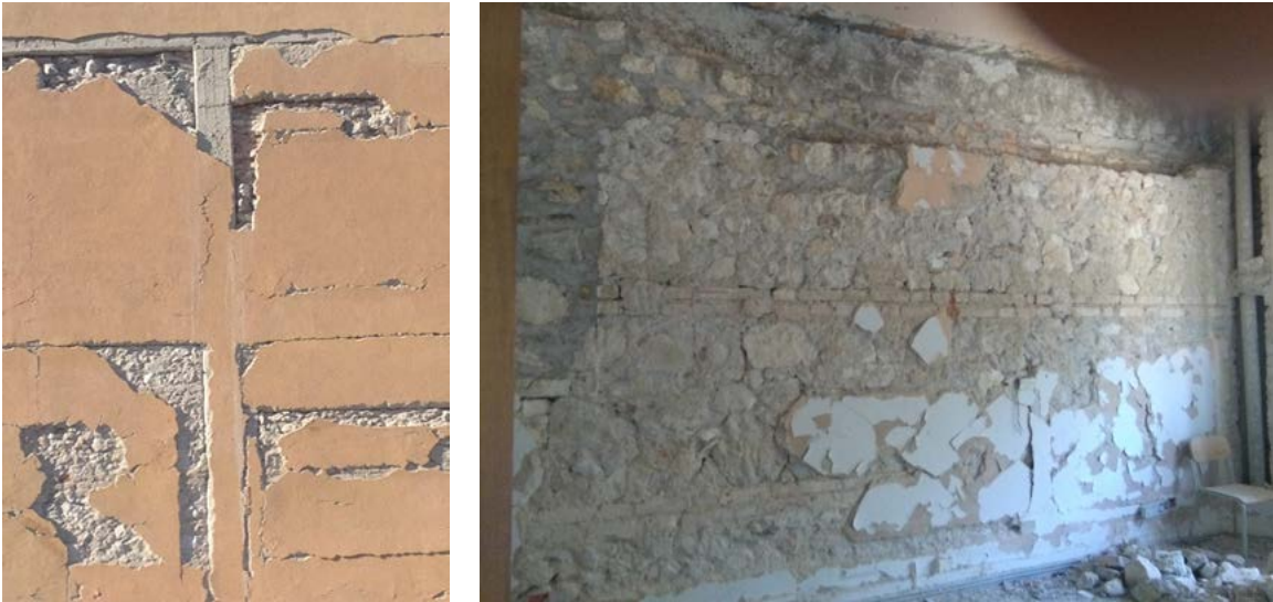
Figures 25-26. Montelucio di Roio, Colony IX Maggio. Exterior and interior details of the walls (photos by S. Ciranna).
