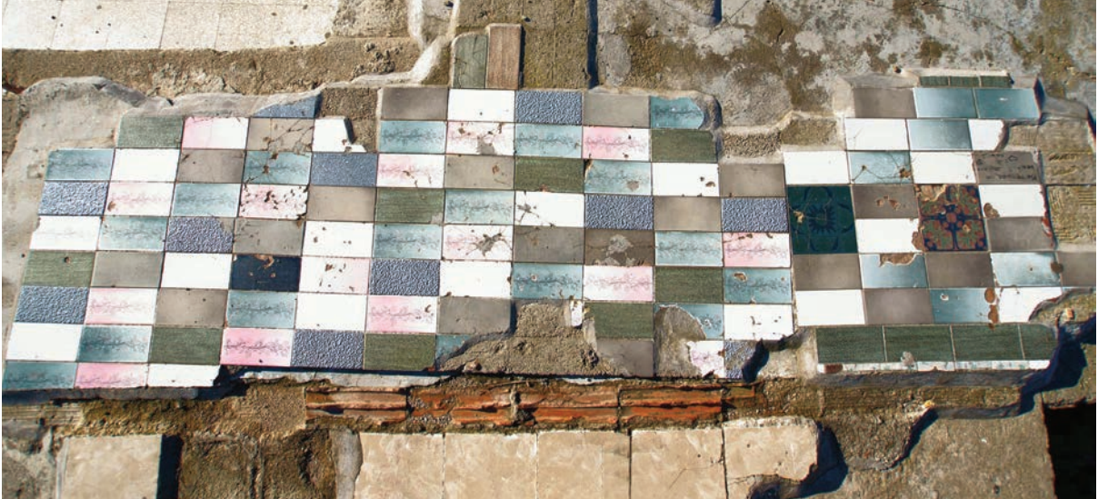
Figure 26. Turó de la Rovira - Barcelona. Views of Els Canons area after the restoration in 2011 (photo by F. Aiello - www.francescoaiellophotographer.com ).
