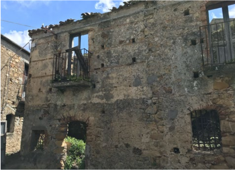
Figure 23. Ferruzzano, Reggio Calabria. The insertion of a portion built after the earthquake of 1908 on a pre-existing undamaged masonry (photo N. Sulfaro, 2022).
