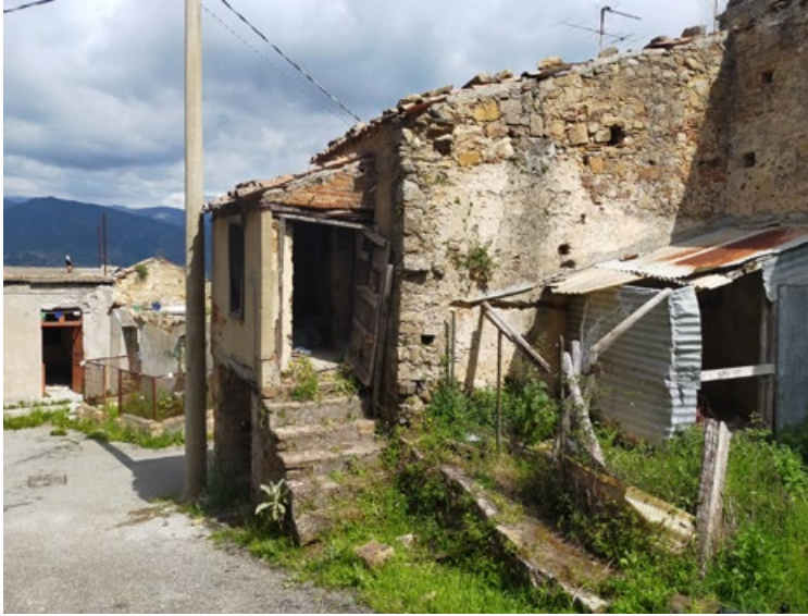
Figure 5. Ferruzzano, Reggio Calabria, pilot project. Addition of external bathroom (unit 324) (photo S. Pistidda, 2023).
